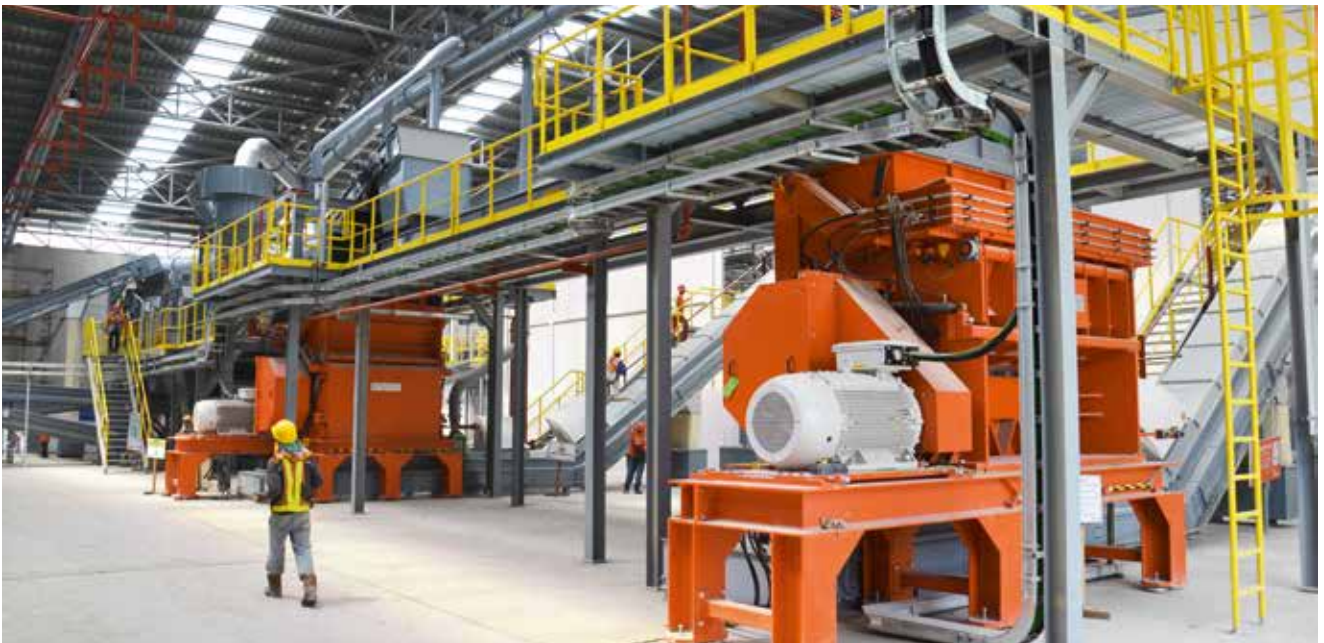
2x FineCut 2500 with power belt drive, Indonesia
